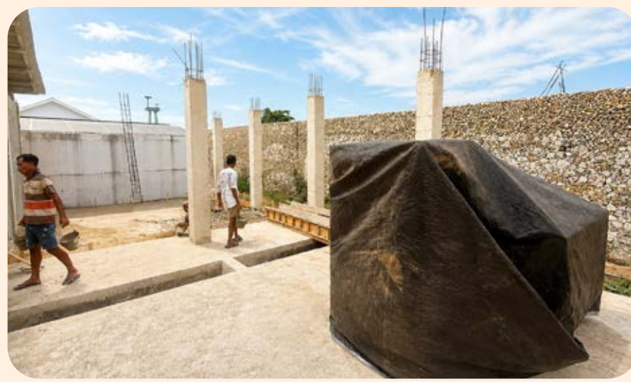
Photo: New trafo and new trafo room
